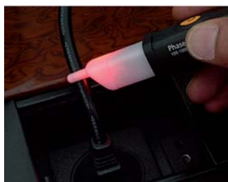
Incorrect phase sequence
