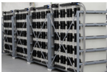
Energy Storage System
